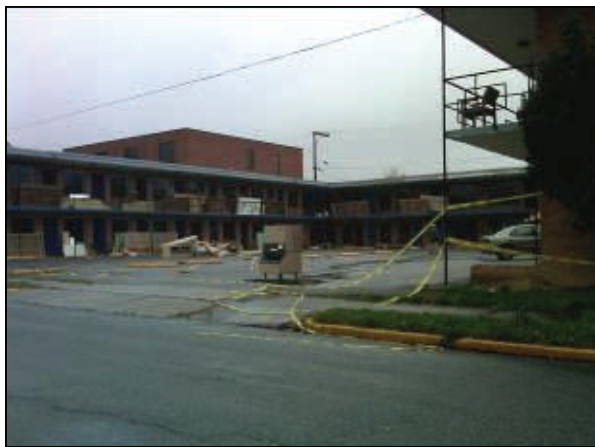
Workers renovate the former Town House Motel. Is this going to be the residence of transient Zachry workers?
